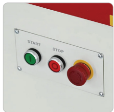
Main Control Panel with Emergency Stop
